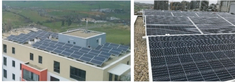
FIGURE 1: The roof type SPP and its PV panels.
